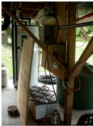
Figure 3. Battery bank at a household using photovoltaic (solar) panels.
